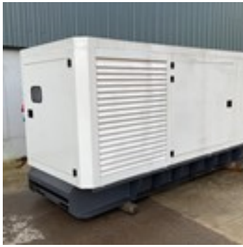
350KVA Ashvale Engineering Generator
